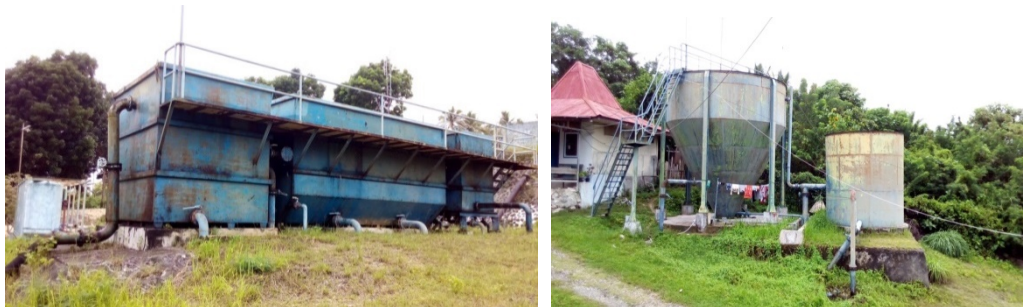
Figure 3. Water Treatment Plants (WTP) of Keles
